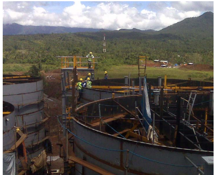
Carbon-in-leach tank train.
