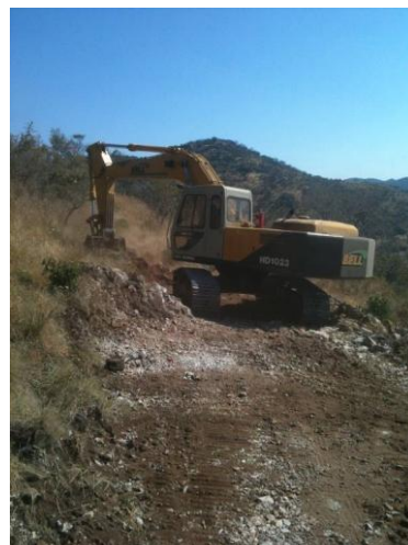
Figure 1 - Excavation of the access road on the hill at Kaskara in preparation for a systematic drill programme of 30 holes.
