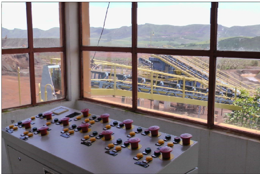
Fig. 4 Processing plant control room
