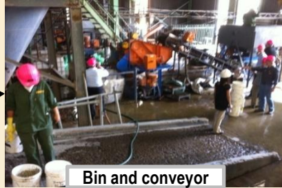
Bin and conveyor
