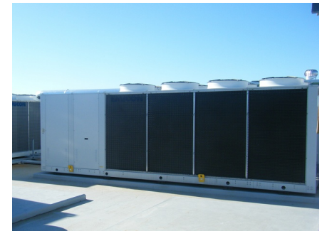
Chiller for Air Conditioners
