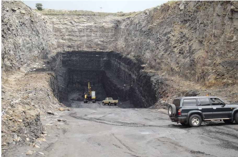
Diagram 2 Overview of box cut excavation showing 18m-thick coal seam below 15m of overburden
