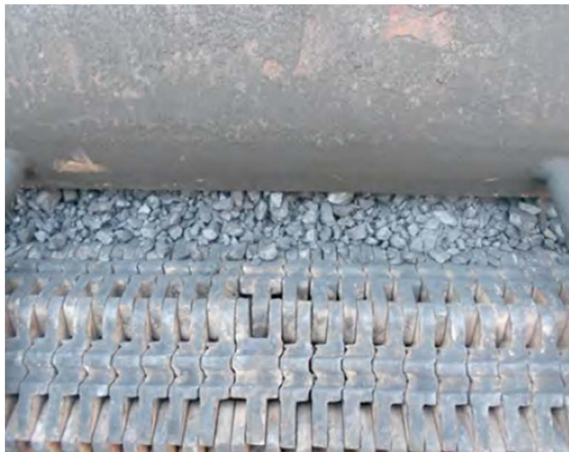
Diagram 2. Sese coal on the bed of the chain-grate feeding into the boiler
