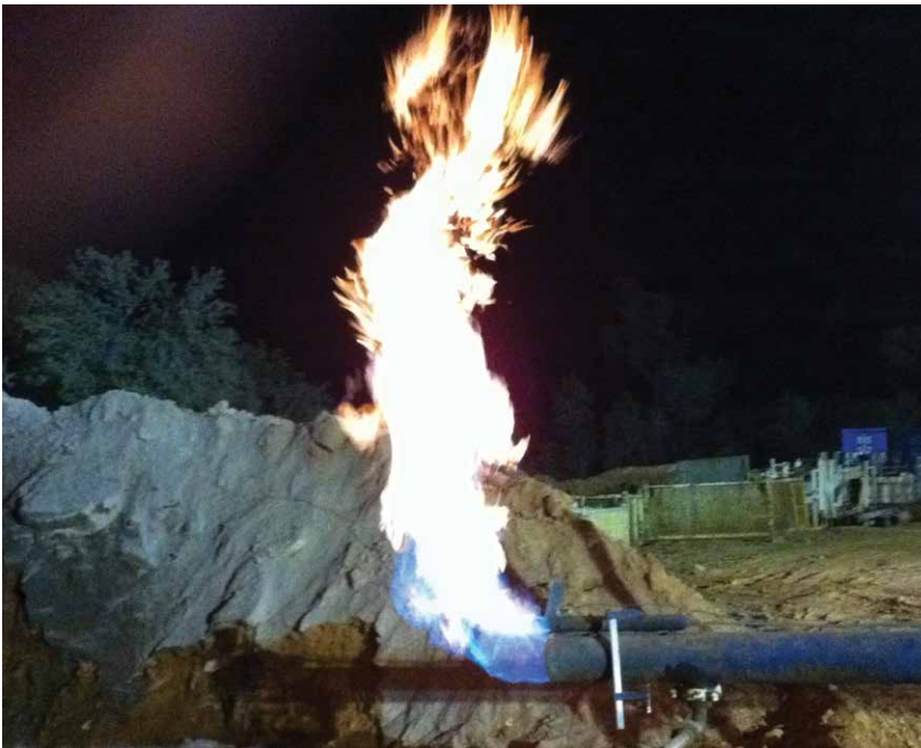
Figure 5 Gas burning from the end of the 8" diameter "blooie" pipeline, venting the Cow Lagoon 1 well
