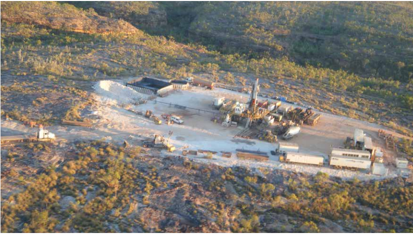
Figure 7 Aerial view of the Glyde1 lateral well site
