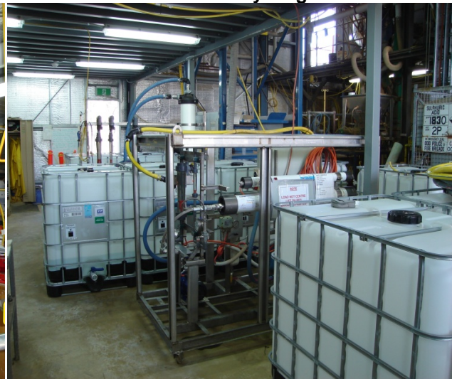
Reverse osmosis water recycling DPP
