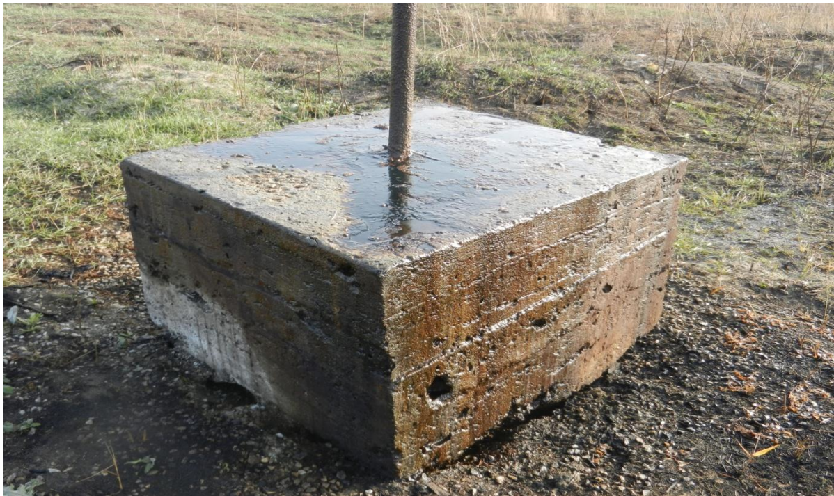
POV- 2 showing Oil Seepage
