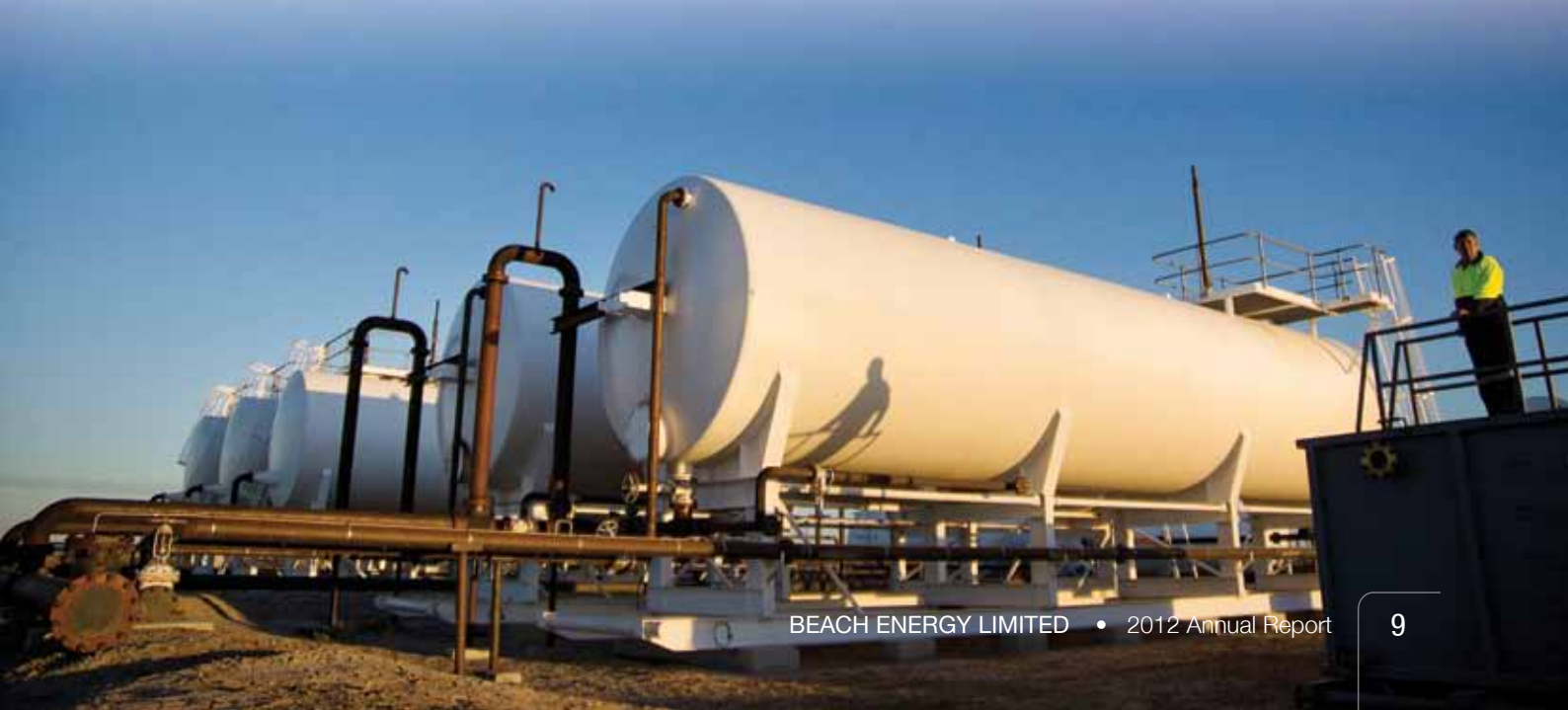
Dewatering tanks at the Callawonga tank farm in PEL 92
