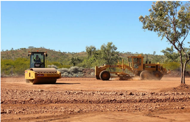
Figure 20: Grader and roller preparing the Administration Building site - all machinery owned 100% by CuDeco
