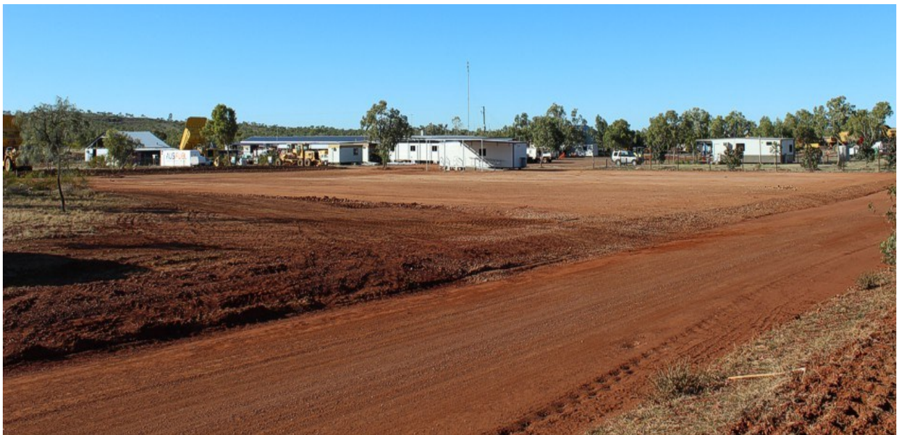
Figure 25: Preparing haul roads (top left); preparing Workshop and Office Complex areas (top right) and; administration buildings area cleared at entry to Rocklands (above) - all machinery owned 100% by CuDeco
