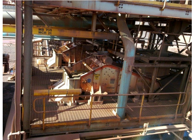
Figure 11: example of Rocklands scale (3mtpa), allmineral alljig® gravity plant at BHP's Whyalla Project, South Australia - alljig® screening plant
