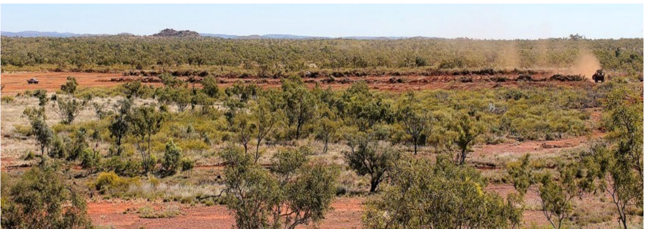
Figure 18: Plant site being cleared and levelled in preparation of major civil works
