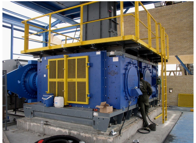
Figure 15: Installation technician working on the hydraulic hosing - recent HPGR installation by Polysius in the Middle East
