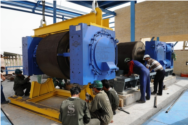
Figure 12: Lifting one of the two Grinding Rolls into position - recent HPGR installation by Polysius in the Middle East
