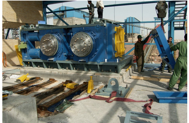
Figure 13: Positioning the HPGR Drive Shafts - recent HPGR installation by Polysius in the Middle East
