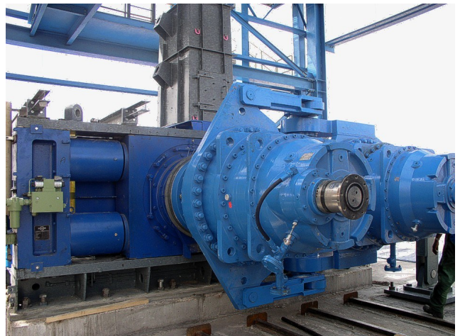
Figure 17: HPGR Hydraulic couplings prior to the drive shaft connections - recent HPGR installation by Polysius in the Middle East
