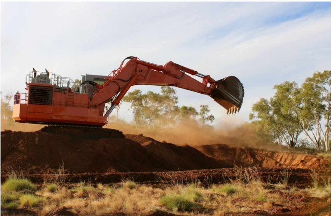
Figure 24: Large scale Hitachi digger removing fill for use as road base - all machinery owned 100% by CuDeco
