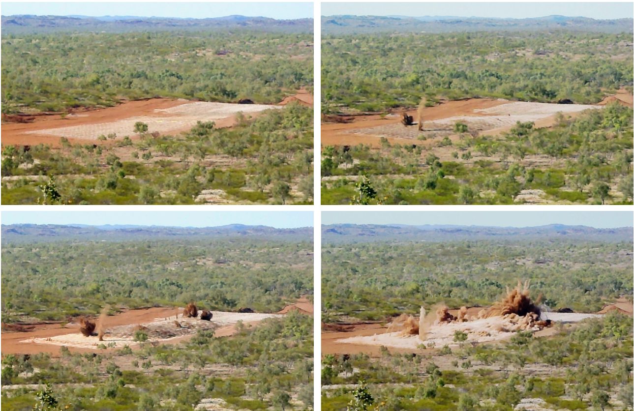
Figure 1: First "shot" of the project...an event long anticipated by all on site who have worked tirelessly on the project through the good times and the tough times, and by the many shareholders who have shared the journey with us. It is an unambiguously significant milestone, and has been a significant journey since the first discovery hole back in 2006.
