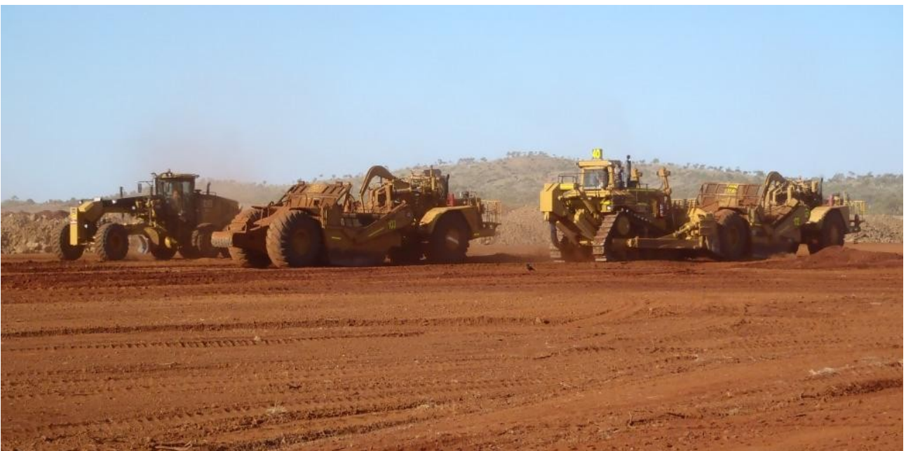
Figure 33: Pre-strip clearing of organic material and topsoil from the Process Plant area
