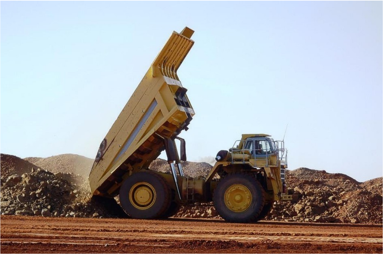
Figure 32: Dump truck unloads rock for use in the Water Storage Facility (WSF) Dam Wall construction.
