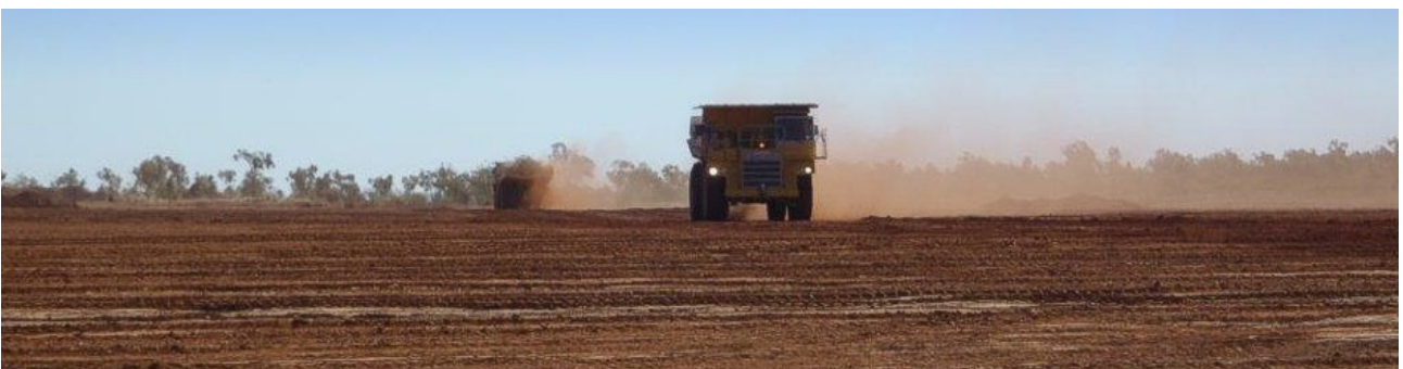
Figure 36: Dump trucks hauling material for use as road base from the mobile crushing plant to various locations on site.
