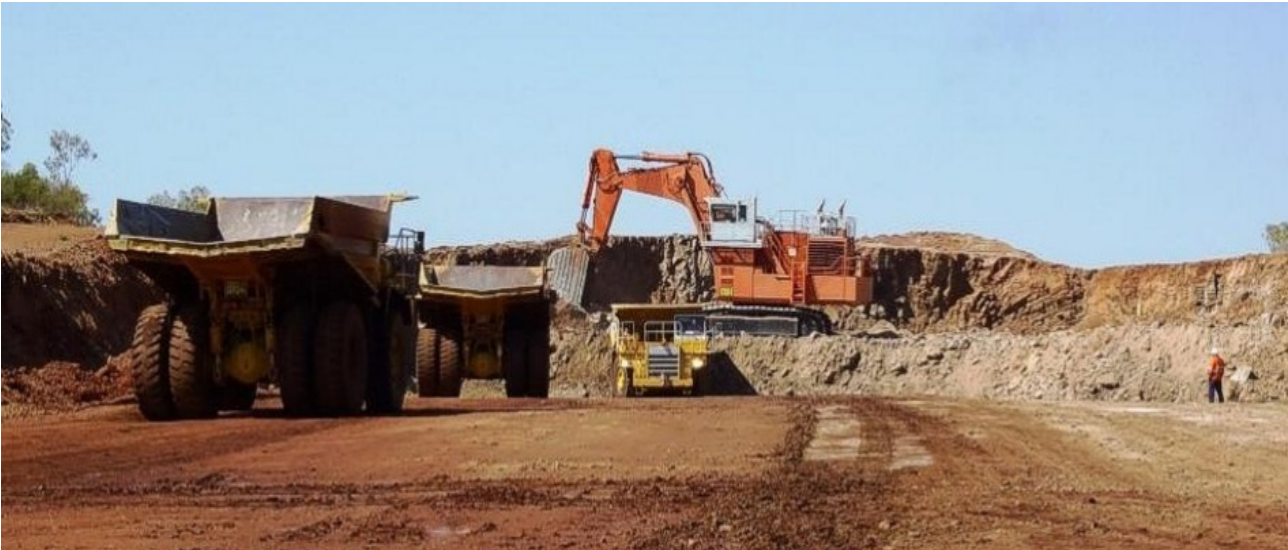
Figure 25: Excavation of a large cutting for the Morris Creek Diversion Channel - anticipated to be completed prior to the onset of the wet-season.
