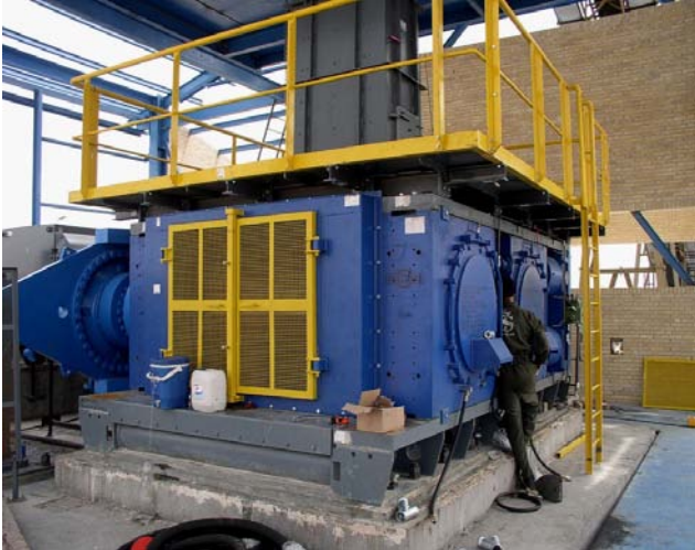
Figure 20: Installation technician working on the hydraulic hosing - recent HPGR installation by Polysius in the Middle East. CuDeco's HPGR will be capable of processing material at the rate of 390 tonnes per hour
