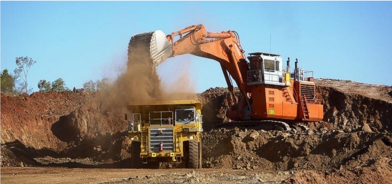
Figure 40: Excavation of a large cutting for the Morris Creek Diversion Channel - anticipated to be completed prior to the onset of the wet-season.
