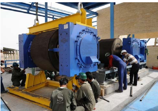
Figure 18: Lifting one of the two Grinding Rolls into position - recent HPGR installation by Polysius in the Middle East
