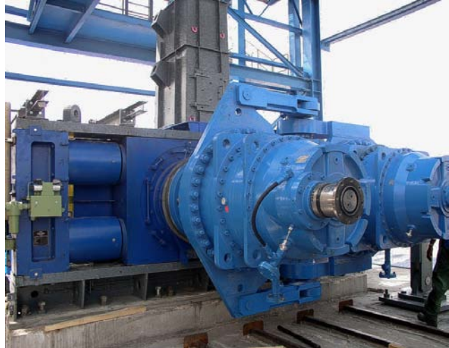
Figure 21: HPGR Hydraulic couplings prior to the drive shaft connections - recent HPGR installation by Polysius in the Middle East
