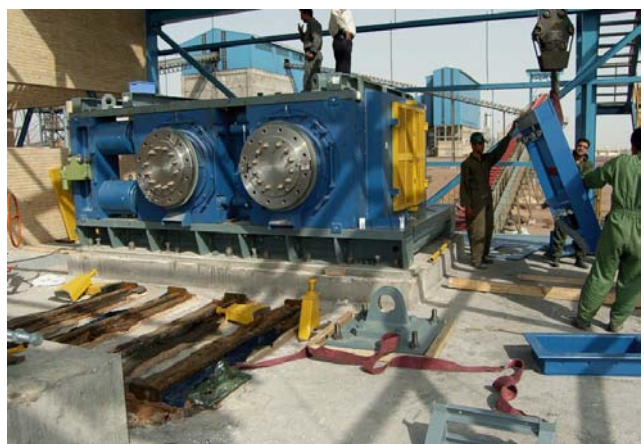
Figure 19: Positioning the HPGR Drive Shafts (2 x 2000hp electric motors) - recent HPGR installation by Polysius in the Middle East. The HPGR pictured is significantly smaller than the one currently being manufactured for the Rocklands native copper circuit
