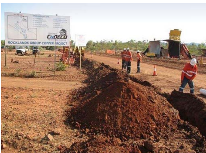
Figure 6: Electrical cable trenching unearths 15m wide copper zone just 1m below surface, beside the Rocklands Group Copper Project sign that greets visitors to the Site Office Complex...literally right under our noses all these years!
