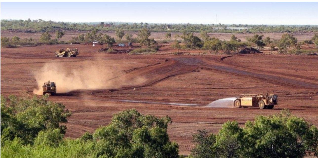
Figure 41: Las Minerale Starter-pit area, being cleared in preparation for initial mining activities. Organic material and topsoil is firstly removed and stored in segregated stockpiles for later rehabilitation, prior to basic pre-mining activities which includes the removal of some areas of surface colluviums. The area cleared for the main Water Storage Facility (WSF) can be seen in the background, behind the intermediate tree-line, and in the far background to the right, the rooflines of the Rocklands Compound...see Figure 3 for approximate pit outline overlay.
