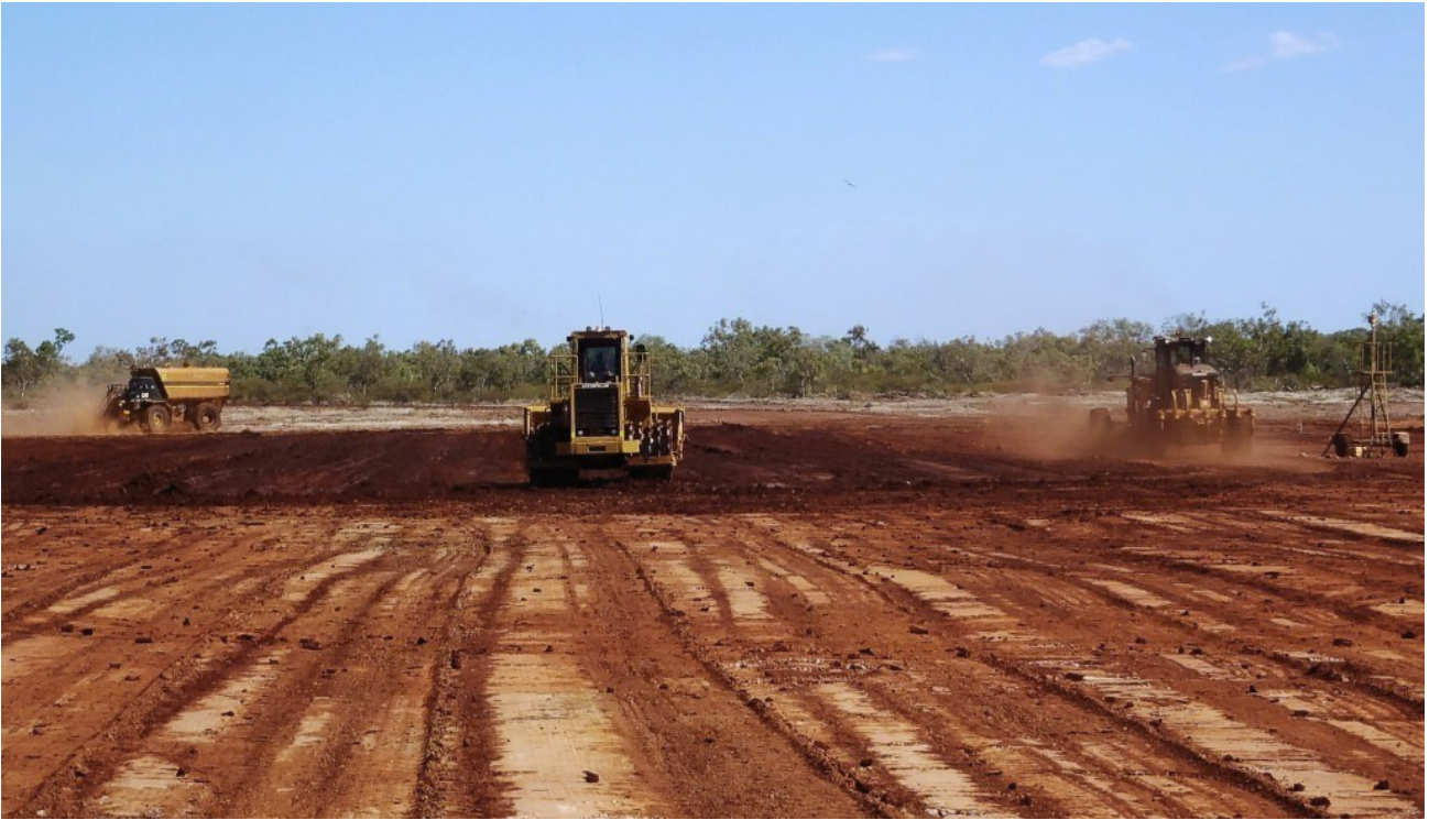
Figure 30: Clearing and preparation of Crusher Pad - foundations and associated concrete work to commence within the week.
