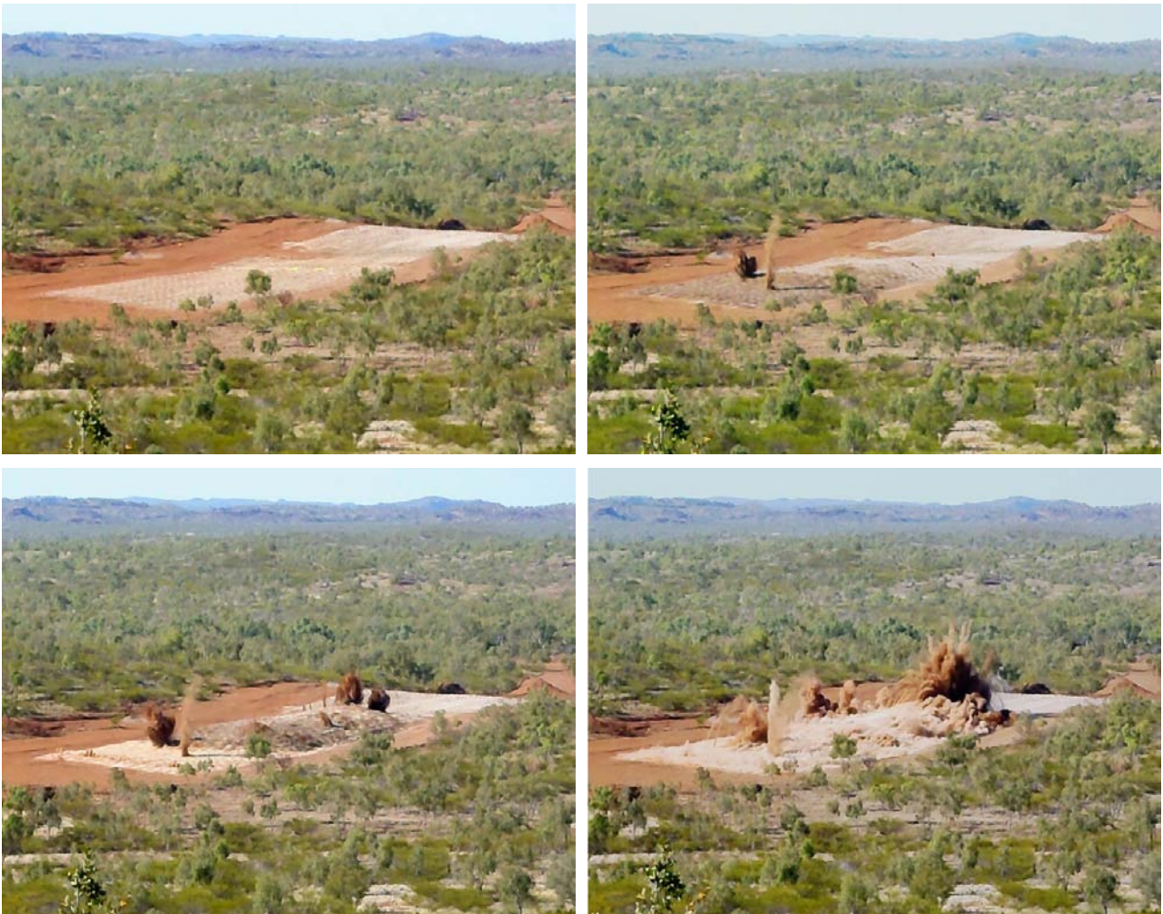
Figure 8: First "shot" of the project...an event long anticipated by all on site who have worked tirelessly on the project through the good times and the tough times, and by the many shareholders who have shared the journey with us. It is an unambiguously significant milestone, and has been a significant journey since the first discovery hole back in 2006.
