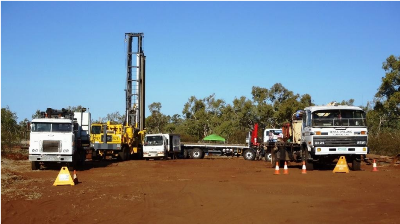
Figure 37: Pit dewatering activities (borehole drilling) - once completed, pumps divert the water to temporary storage facilities distributed throughout Rocklands for use in development works and will eventually be pumped to the WSF once it has been completed.
