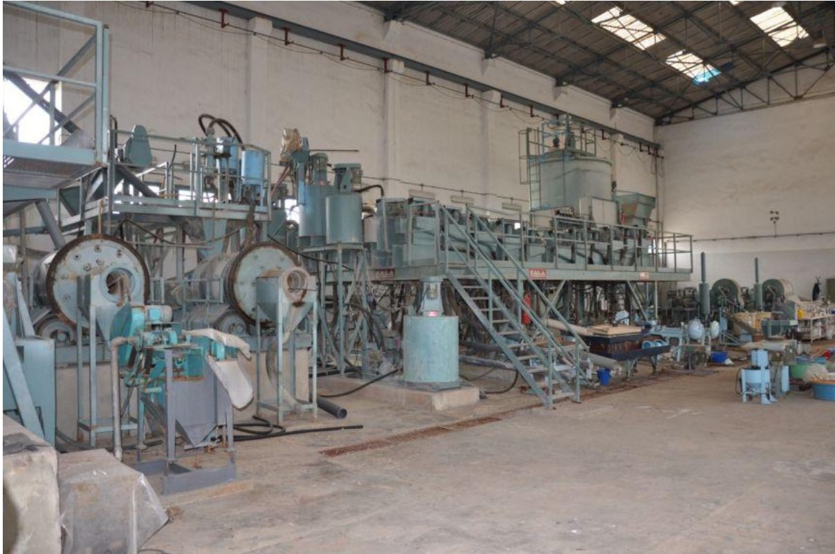
Figure 6 Pilot Plant for Phosphate in Tunisia – Allowing Batch Testing
