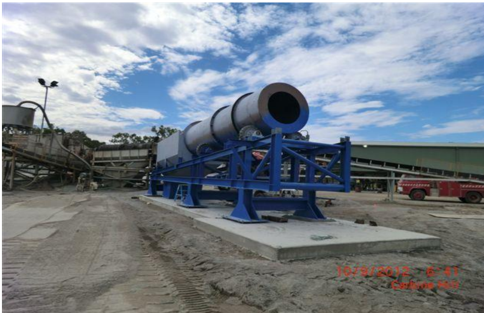
New front end scrubber equipment being installed at CNQ's Mt Carbine Tailings Re-treatment Plant minimising requirements for plant shut-down duration.
