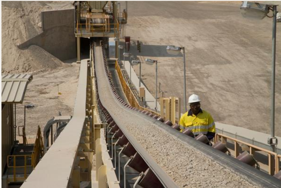
Crushed Ore moving to the Ball Mill
