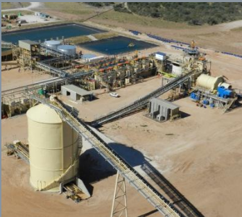
Crushed ore bin and flotation circuit
