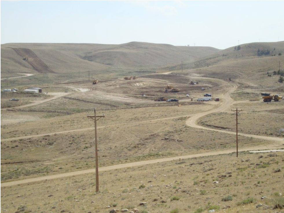
Earth works at the Grieve facility site after removal of original processing facilities
