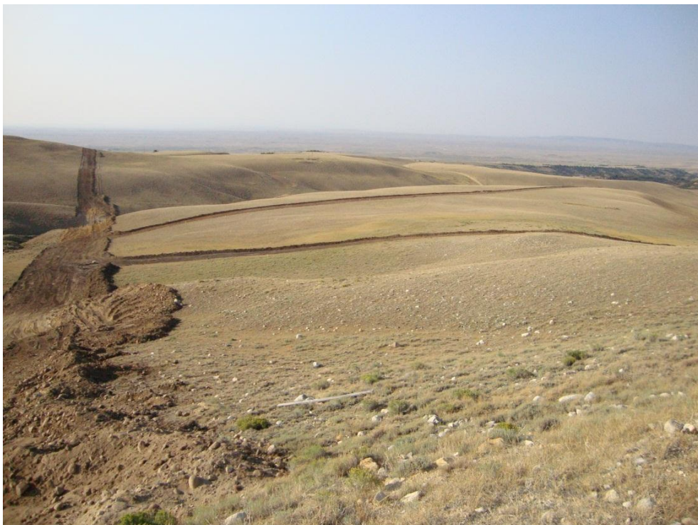
Preparation of the right of way for the laying of Grieve in-field piping
