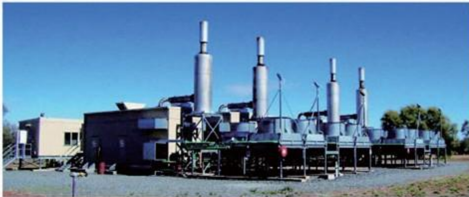
Alice Springs Power Plant, Australia
