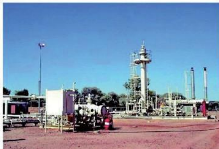
Gilmore Gas Plant, Australia
