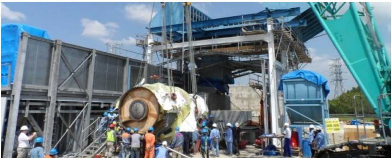
Installation of gas turbine for the Sengkang Power Plant 120MW Expansion Project
