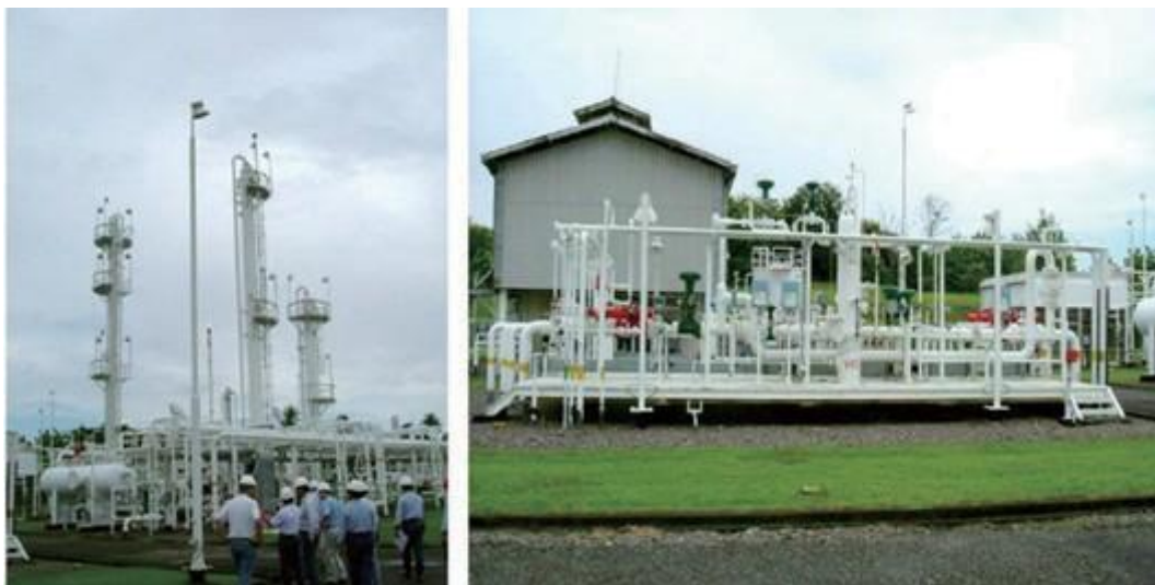
EEES Kampung Baru Sengkang, Indonesia Central Processing Plant (CPP)
