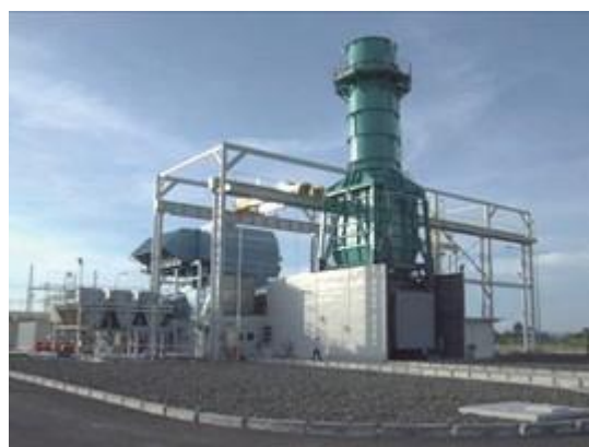
Sengkang Power Plant, South Sulawesi Indonesia first 60 MW expansion (2008)
