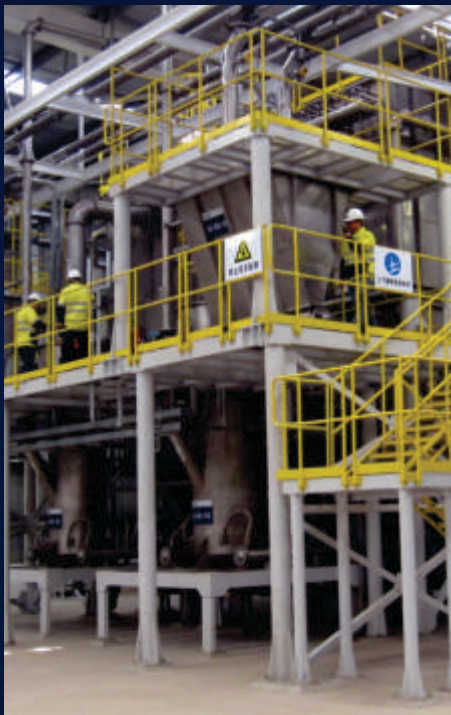
Microniser plant at Jiangsu
