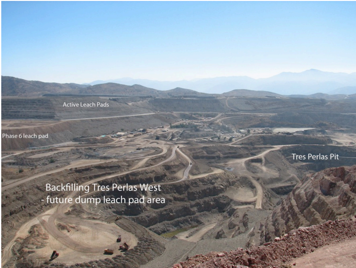
Figure 8 – Backfill of Tres Perlas West Pit For Construction of ROM Leach pad (in foreground)
