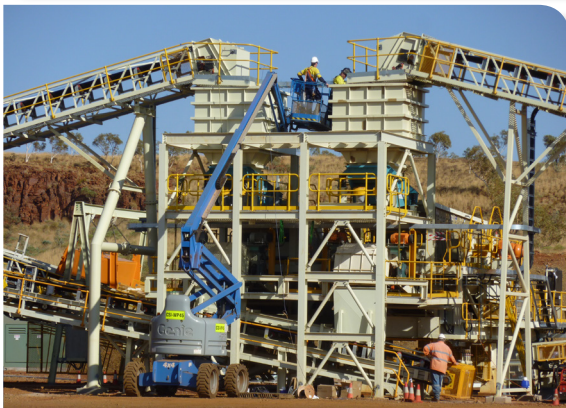
Crushing Services International fitters installing wear liners into the discharge chute of CV2
