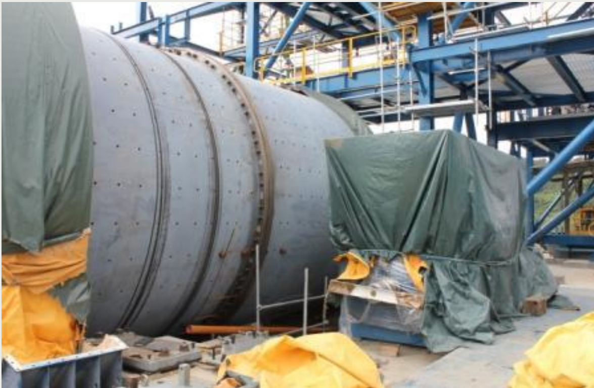
Image 2: Grinding mill motors installed, August 2012
