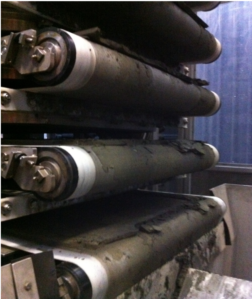
Figure 3 – Concentrate Filter Press at Didipio
