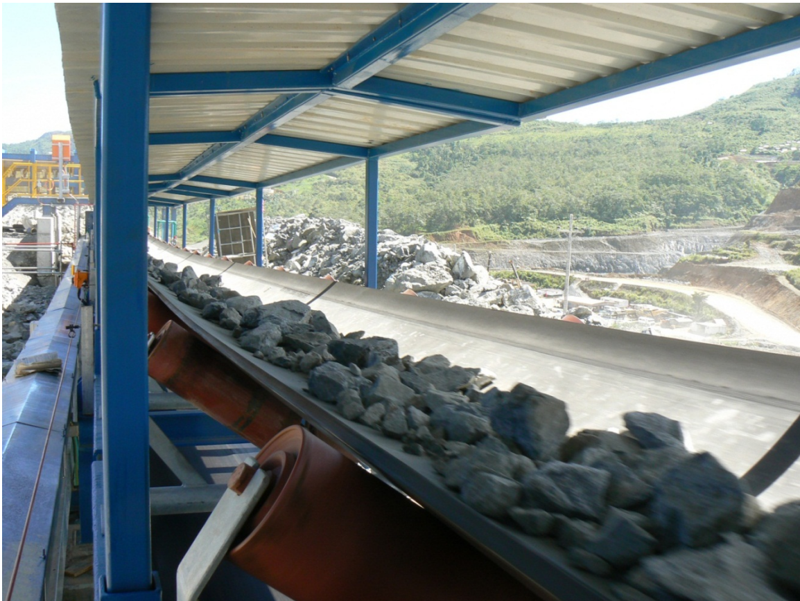
Figure 1 – Commissioning the Conveying System
