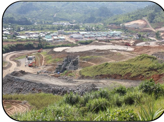
Primary crusher, conveyor & ROM pad
