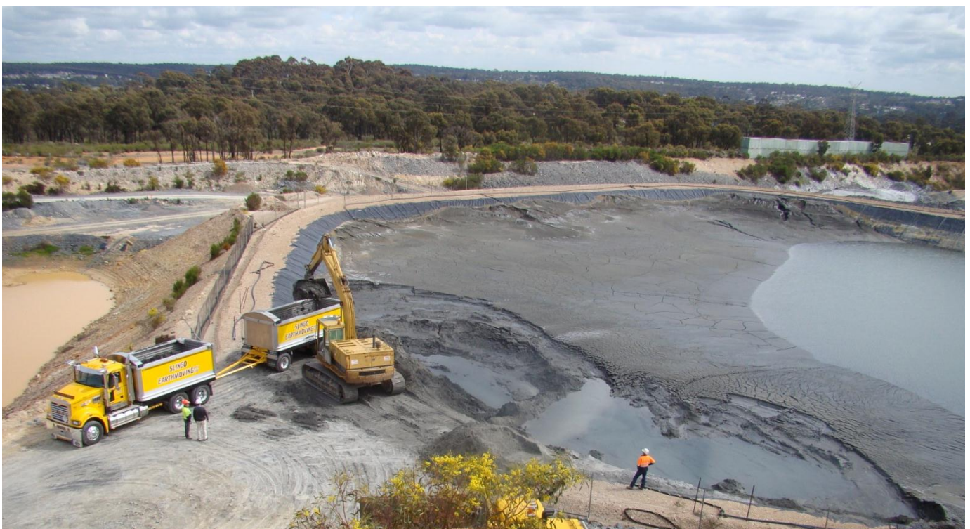
Excavator removing tailings from the flotation concentrate tailings dam at the Kangaroo Flat Gold Mine
