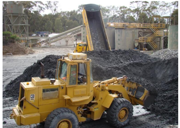
Tailings delivered to the Porcupine Flat Gold Processing Plant
