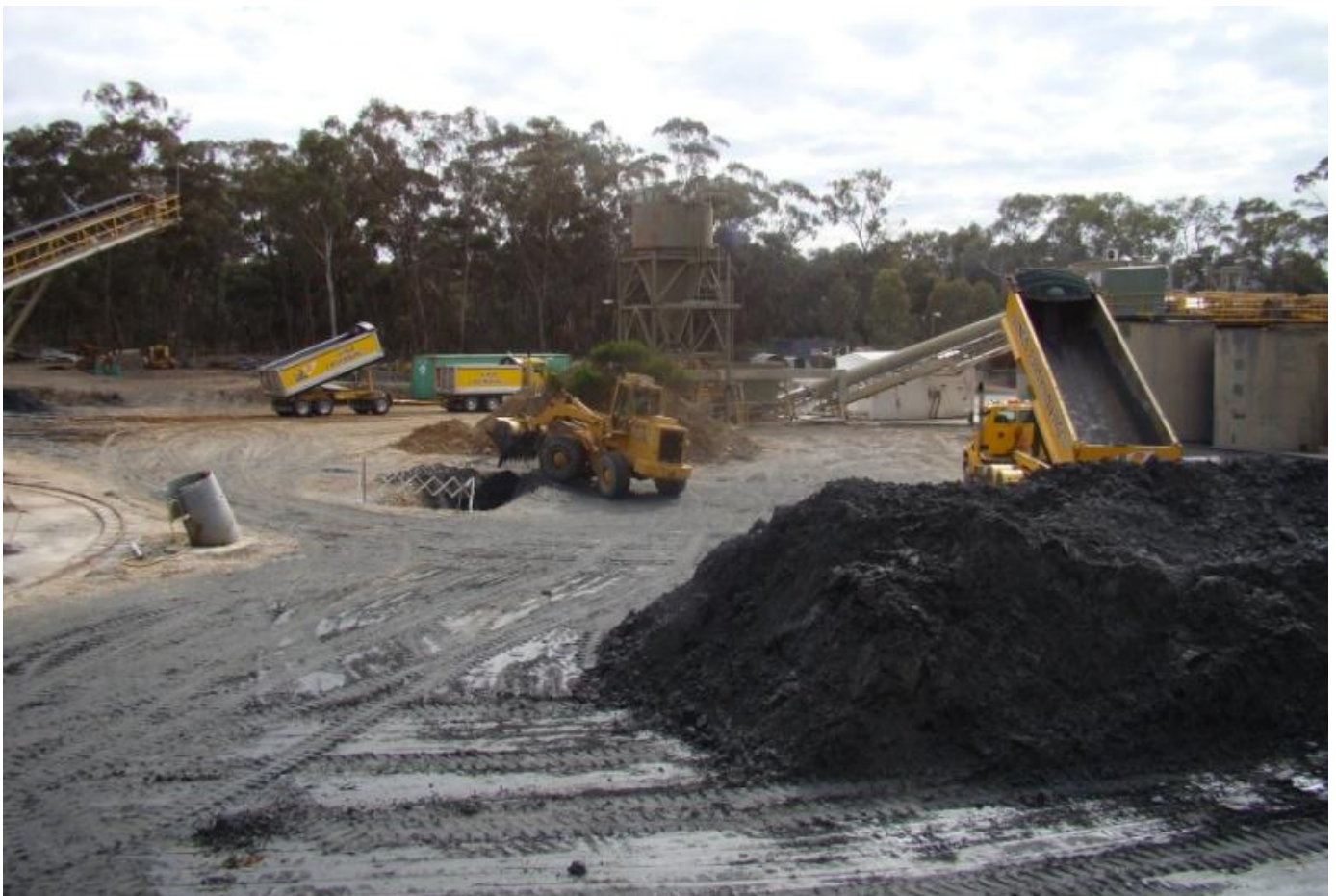
Kangaroo Flat tailings being delivered to the Porcupine Flat Gold Processing Plant with front end loader feeding the ore chute
