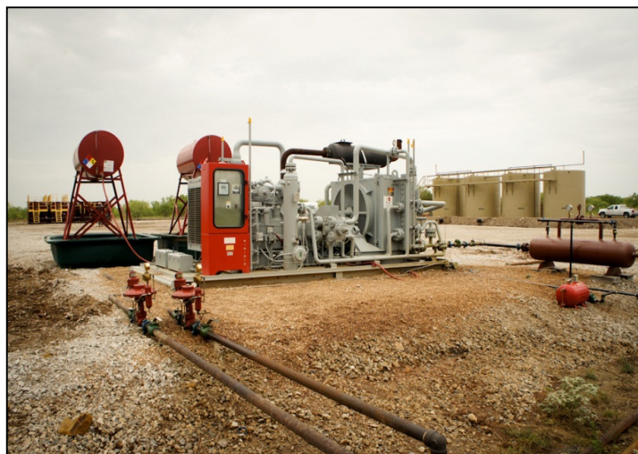
Figure 1; Comanche # 2 Test Well Production Facilities
