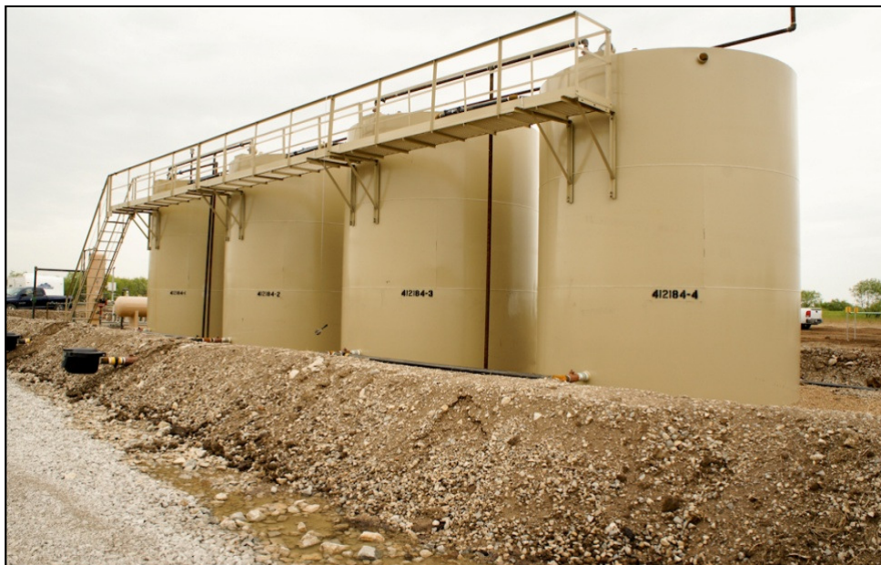
Figure 2: Comanche Test Well #2 Production Facilities
