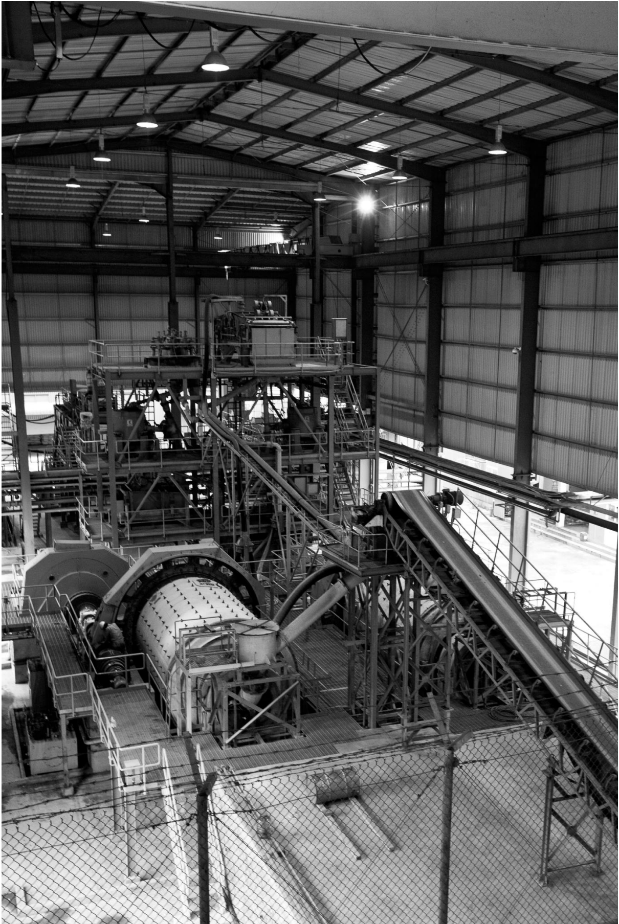
Gold Processing Plant – Phuoc Son, Vietnam
