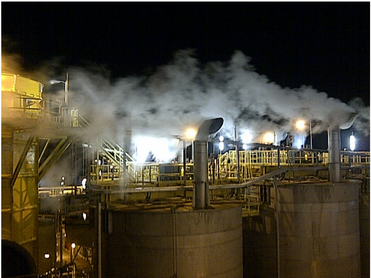
Steam and vapour from oxidation reaction in Albion tanks, and cooling tower
