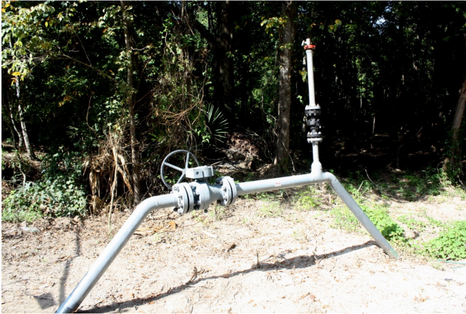
Natural gas tap facilities into main gas sales trunk line
