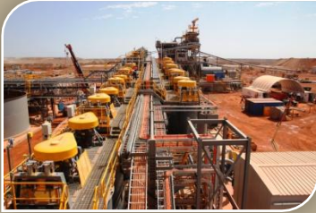
View of the Flotation cells at the 1.5Mtpa DeGrussa processing plant
