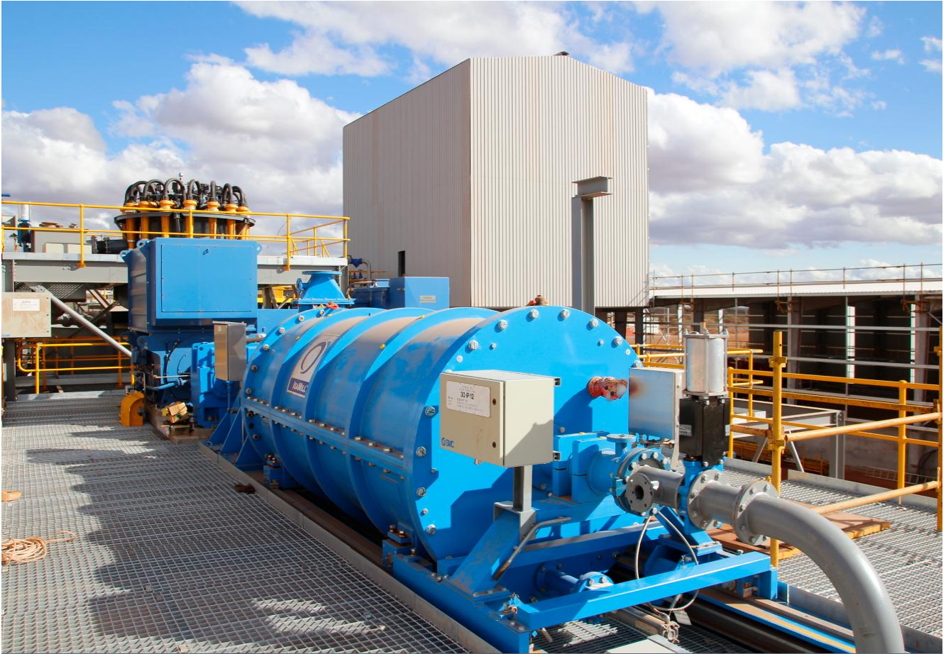
Regrind mill, cyclones and filter building
