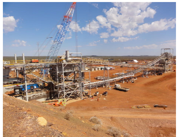
Crushing & Screening plant.
