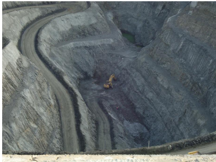
Tim King open pit looking north showing an excavator digging the final cut
