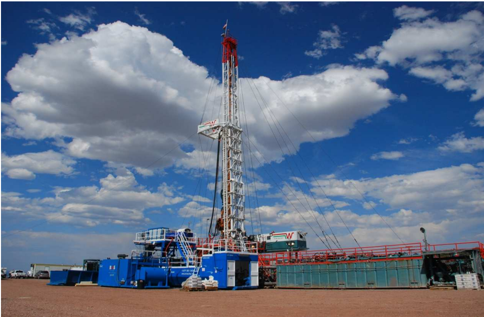
Les Wilson Rig # 30. Drilling at the Company's Pathfinder project underway in Colorado
