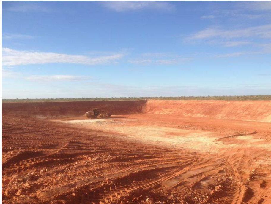
Figure 3. Tailings processing facility for Trial Mining.
