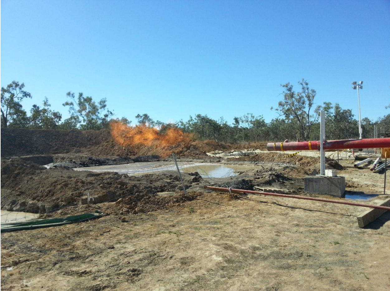
Figure 3 - Eight metre long burning gas flare from gas show at 1098 metres in Armours Egilabria 2 well, ATP 1087 North Queensland.
