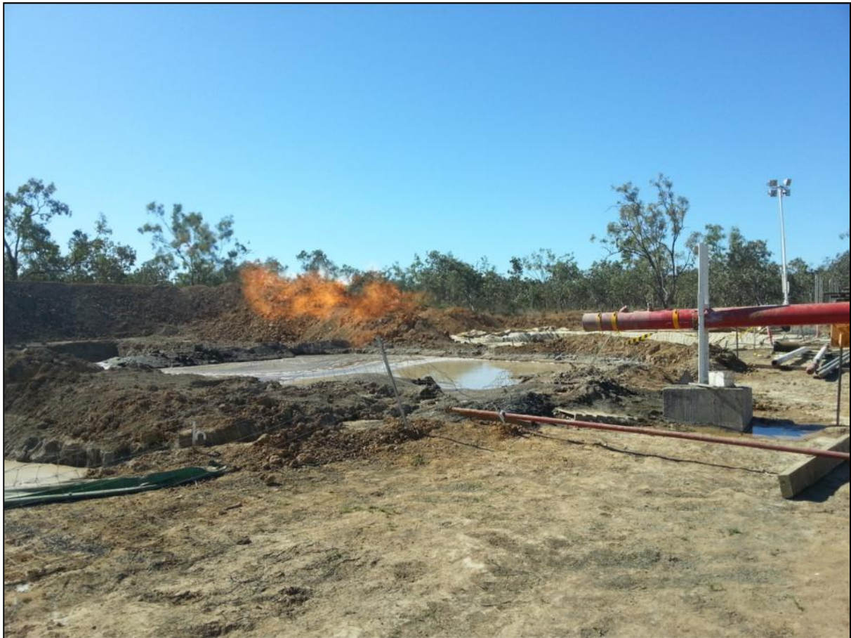
Figure 12: Eight metre long burning gas flare from gas show at 1098 metres in Armour’s Egilabria 2 well, ATP 1087 North Queensland.
