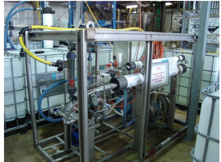
Reverse osmosis and water recycle
