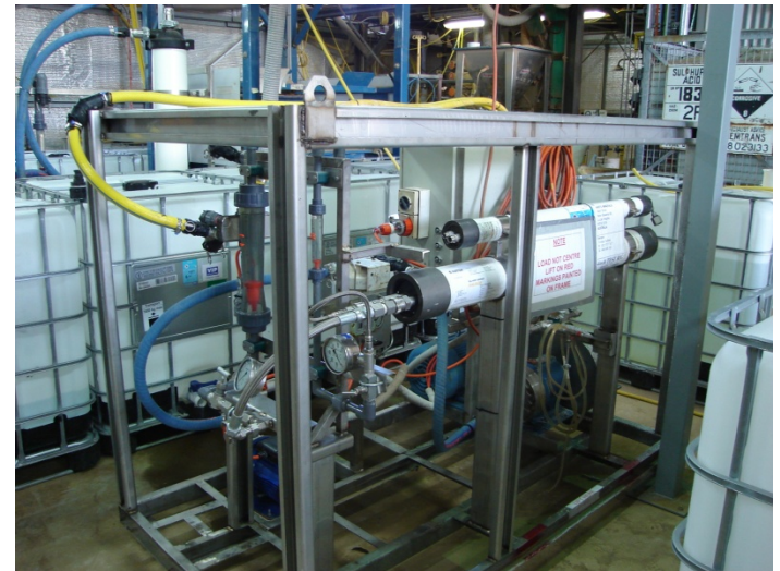
Reverse osmosis and water recycle
