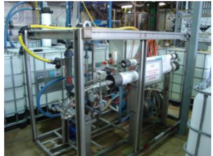
Reverse osmosis and water recycle
