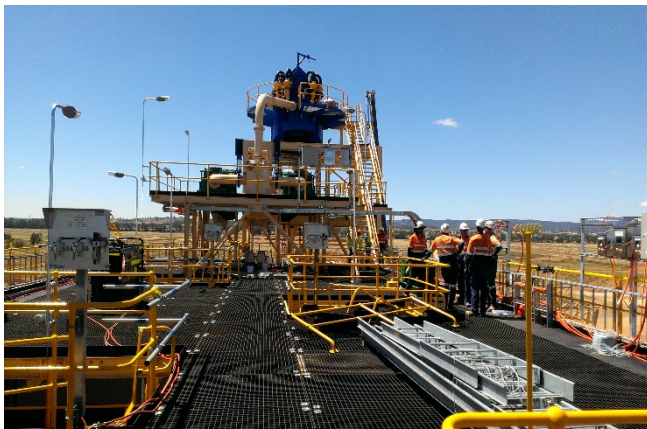
Cyclone circuit on top of CIL tanks
