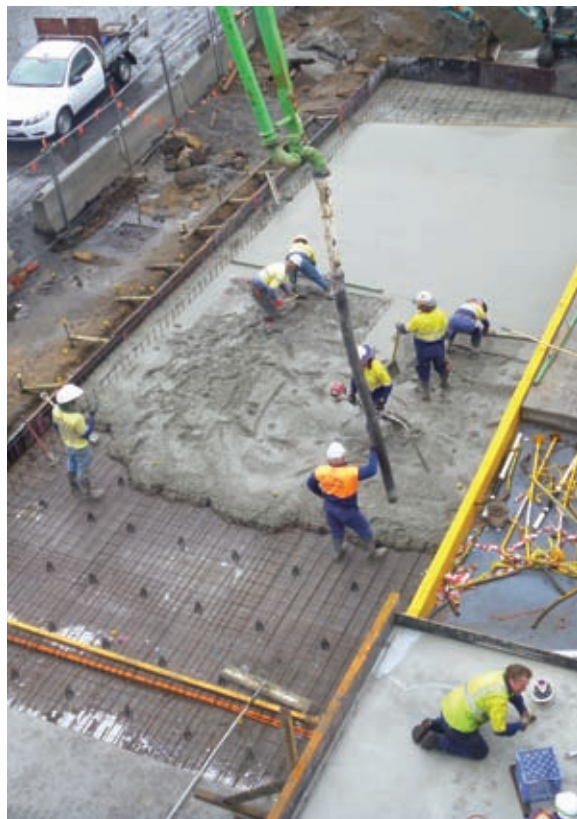
Pouring the slab for the bunded pickle liquor delivery and regenerated acid load-out area
