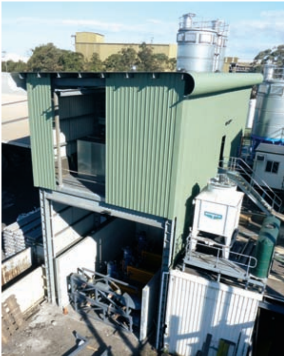
The Plant services room is above the briquetter and the iron briquette load-out bunker. The cooling tower and the holding tank for recycled water are on the right
