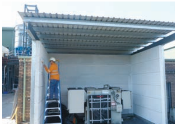
The installation of the 2,000A, 33 kVA transformer and bunded housing is complete
