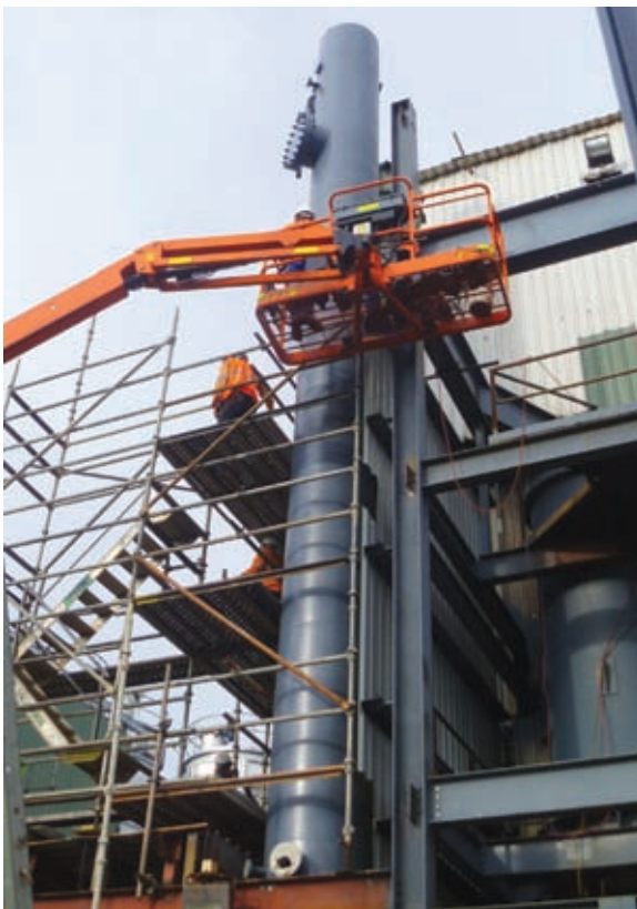
Preparing to install internal fittings into the CO 2 stripping and absorption columns
