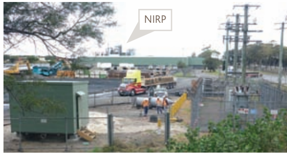
The 33 kVA switchyard and the high voltage switch room which is connected to the NIRP via a 350m underground cable
