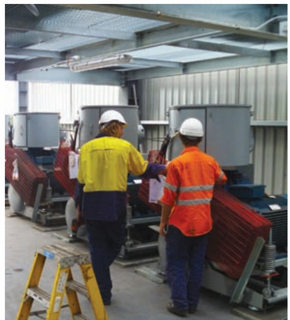
Electrical connection of the blowers on the lower floor of the plant room is underway
