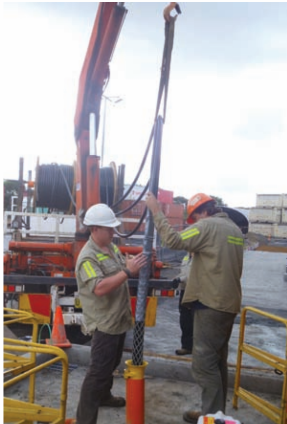
Drawing the cables from the HV transformer to the HV switch room for the 33 kVA power supply
