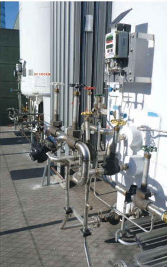
The bulk nitrogen and oxygen storage tanks are now connected to the Plant services room
