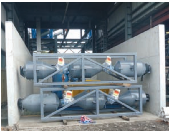
The completed iron briquette load-out bunker is being used to store lock hoppers for the coal delivery system
