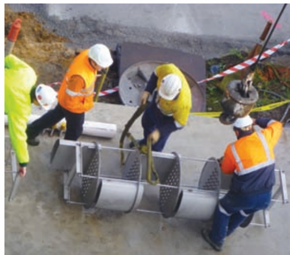
Preparing the internal stainless steel trays for hoisting. The trays facilitate gas-liquid contact and achieve gas absorption in the columns
