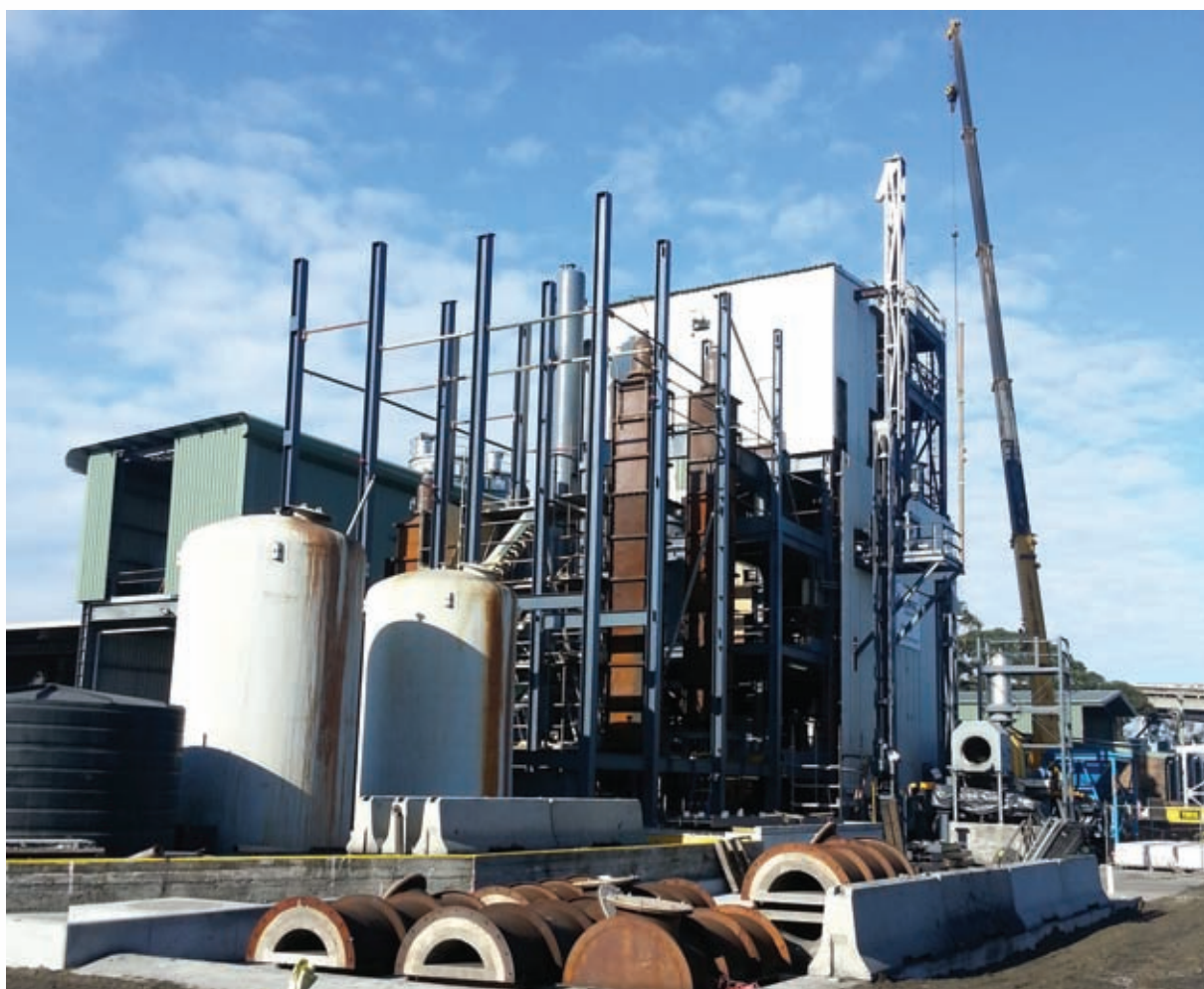
View of the Plant from the northwest, showing the mill scale handling section on the western wall, the structural steel for the north tower extension with the stove shells in position, the stove front covers stored in the completed bunded tanker delivery area (foreground), and the completed Plant services room (upper left centre)
