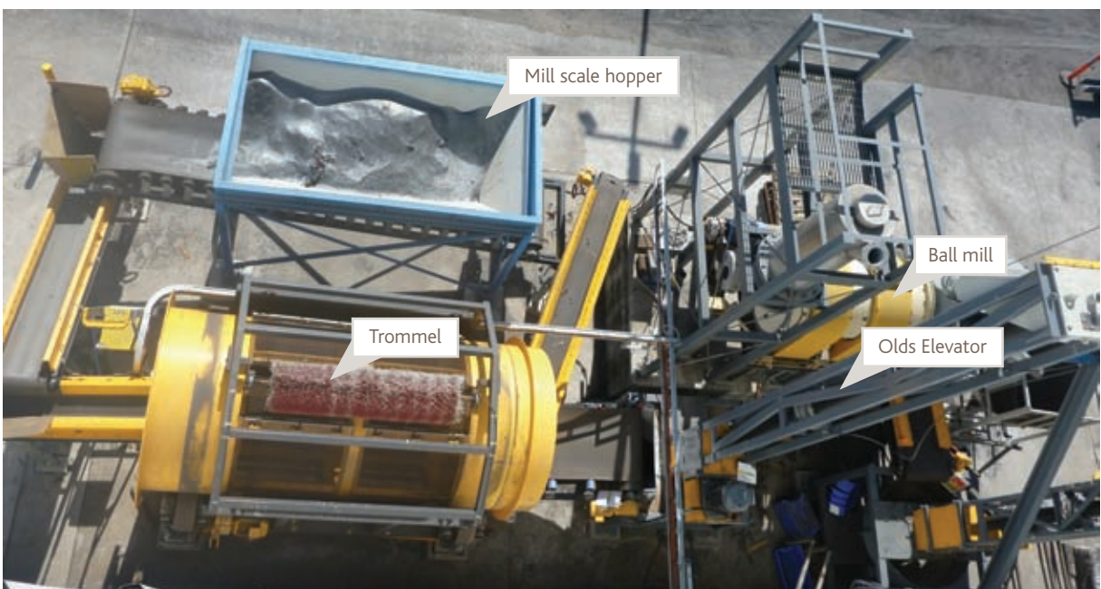
Birds-eye view of the mill scale handling section of the Plant. Raw mill scale will be conveyed from the hopper to the trommel screen, then via an Olds elevator to the ball mill, preparatory to being elevated into the evaporation section in the Plant
