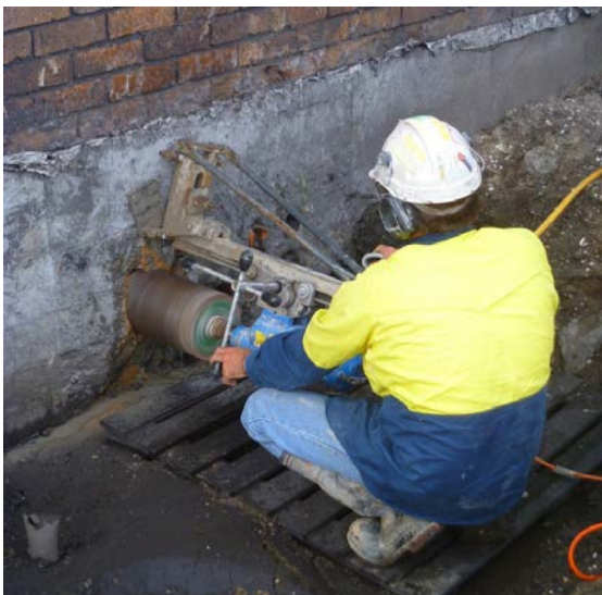
Diamond drilling through foundations to establish cable access to the switch room
