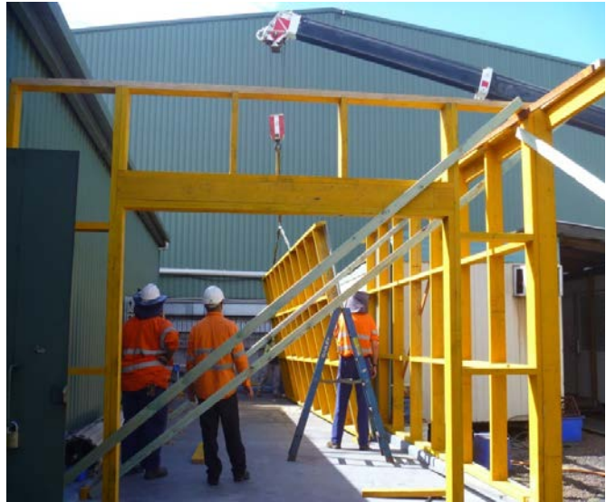
Erection of walls for the new laboratory. Pilot scale test equipment will be relocated from the NIRP process tower and installed here
