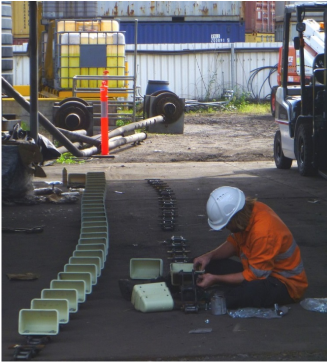
Assembling the bucket elevator chain used to transfer the briquetted iron product
