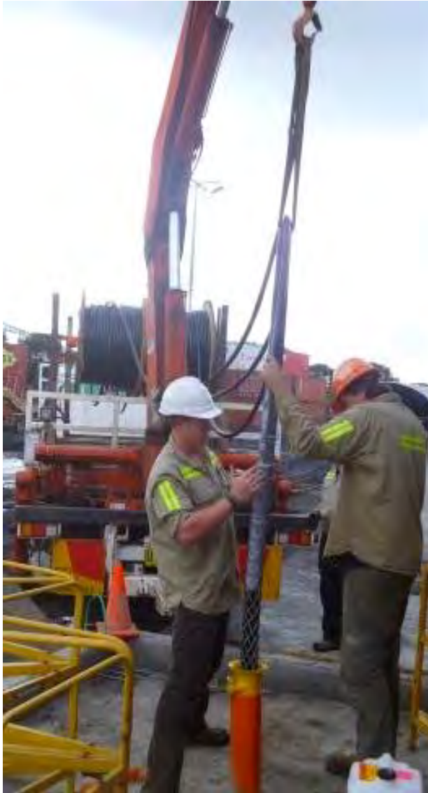
Drawing the 33 kVA cables from the HV transformer to the HV switch room
