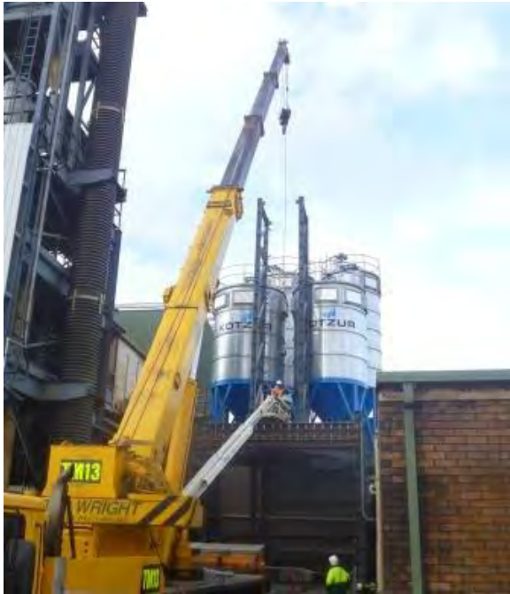
Installing the lower section of the tower to support the magnetic separator (to separate iron chips from char before the products are diverted to their respective silos)
