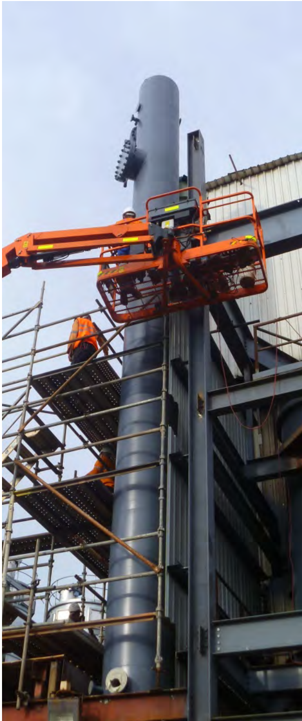
Preparing to install internal fittings into the CO 2 stripping and absorption columns
