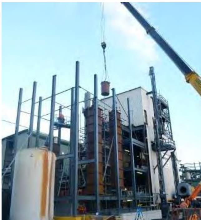
Hoisting the fibreglass tank which will hold strong acid into the north tower
