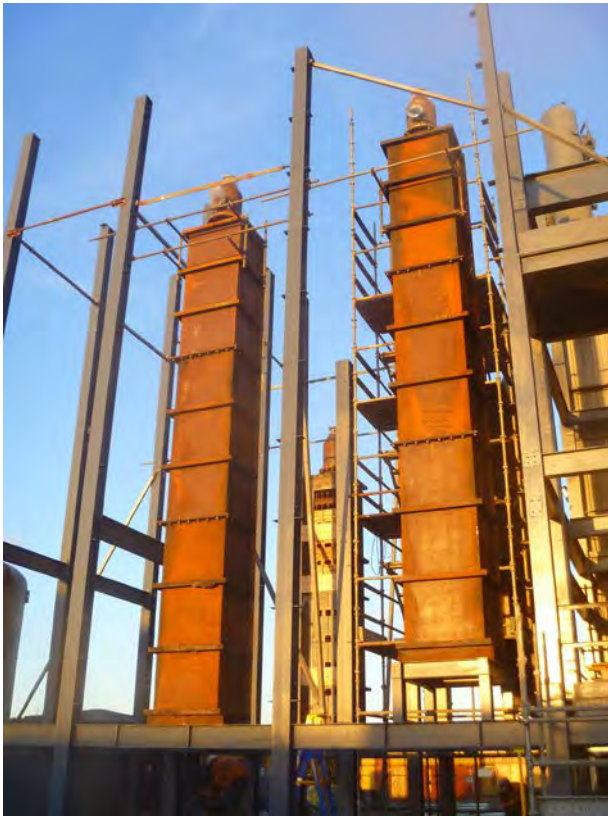
The four stoves for heat recovery and transfer have been installed in the north tower
