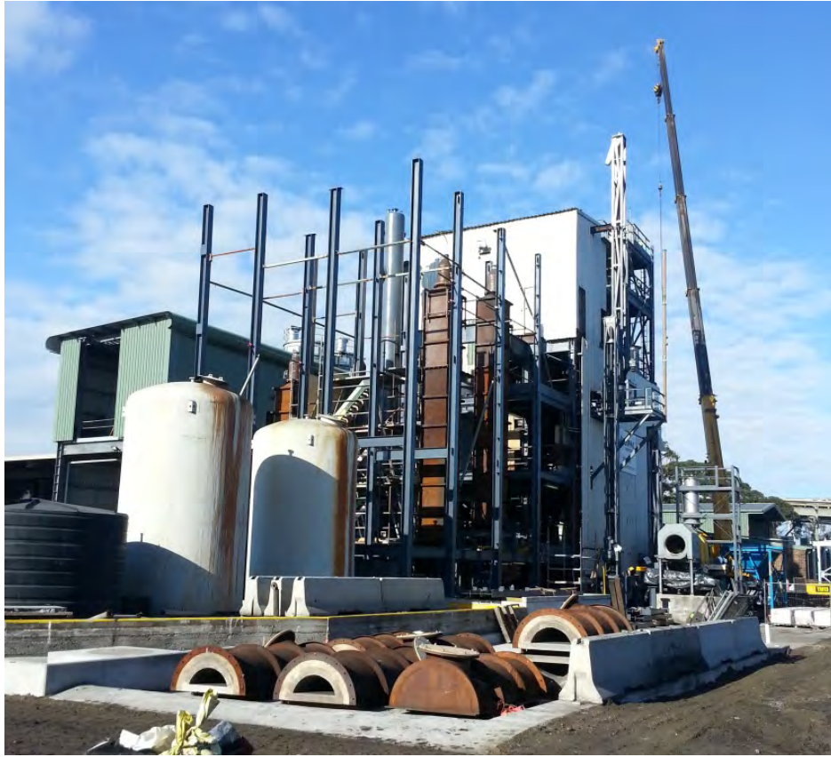
View of the Plant from the north-west, showing the mill scale handling section on the western wall, the structural steel for the north tower extension with the stove shells in position, the stove front covers (foreground), and the completed plant room (upper left centre)
