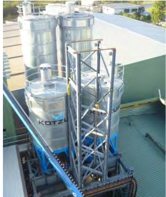
The completed lower section of the tower. The two silos in the foreground will store iron chips (right) and char (left)
