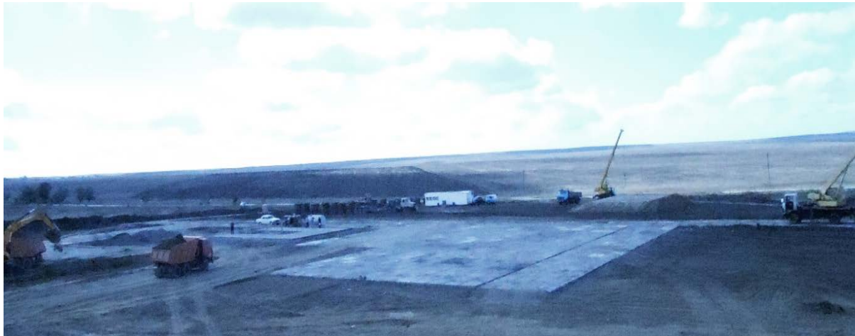
Drill Site and infrastructure is complete and ready to accept the Drilling Rig
