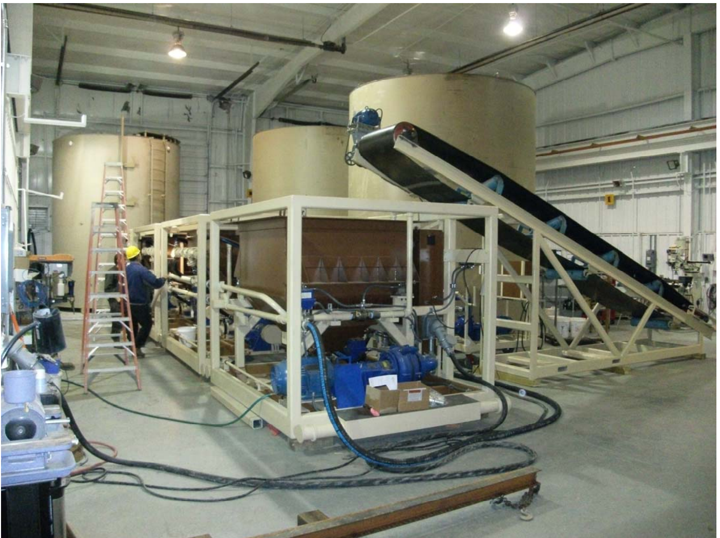
The 5tph Unit during tests in Casper, Wyoming, USA. The slurry mix tank, being fed by a conveyor, is in the foreground. Three interconnected ablation modules are positioned immediately behind the mix tank. Three water storage tanks are evident in the background.
